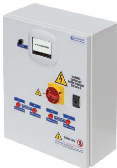
Electric switchboard control for two three-phase unit (tot.240.000 btu) with additional for double pumps.
